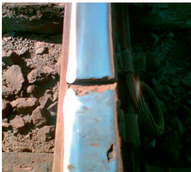
Fig. 1 Metal chipping in the receiving rail within the joint area at one of Transsib track sections (passed tonnage is 420.2 million tons)
