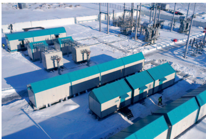
Traction substation 110/27.5 /10/3.3kV at Engels locomotive-building plant
