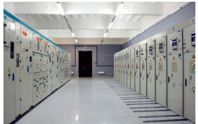
DC switchgear 3.3 kV and AC switchgear 10 kV at traction substation on the St. Petersburg - Buslovskaya section of the Oktyabrskaya Railway
